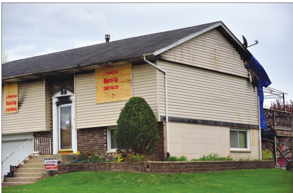
Fire-damaged home in the 700 block of Lacy Avenue.
